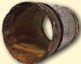
Anodes protect plumbing
